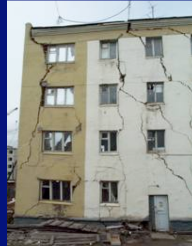
Foundation Settling in Chersky
